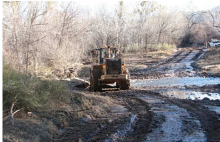
Pinal County heavy machinery caught in action, illegally blading a road across the San Pedro River in designated Critical Habitat for the federally endangered Southwestern Willow Flycatcher.
