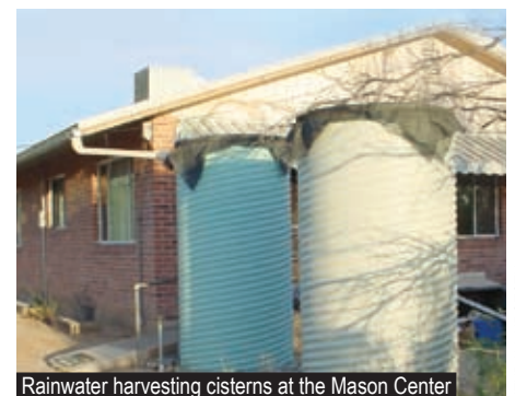
Rainwater harvesting cisterns at the Mason Center
